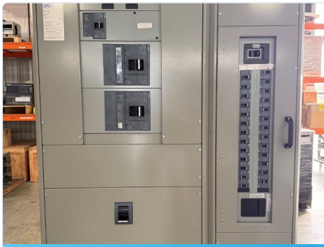
MAIN DISTRIBUTION SECTION
